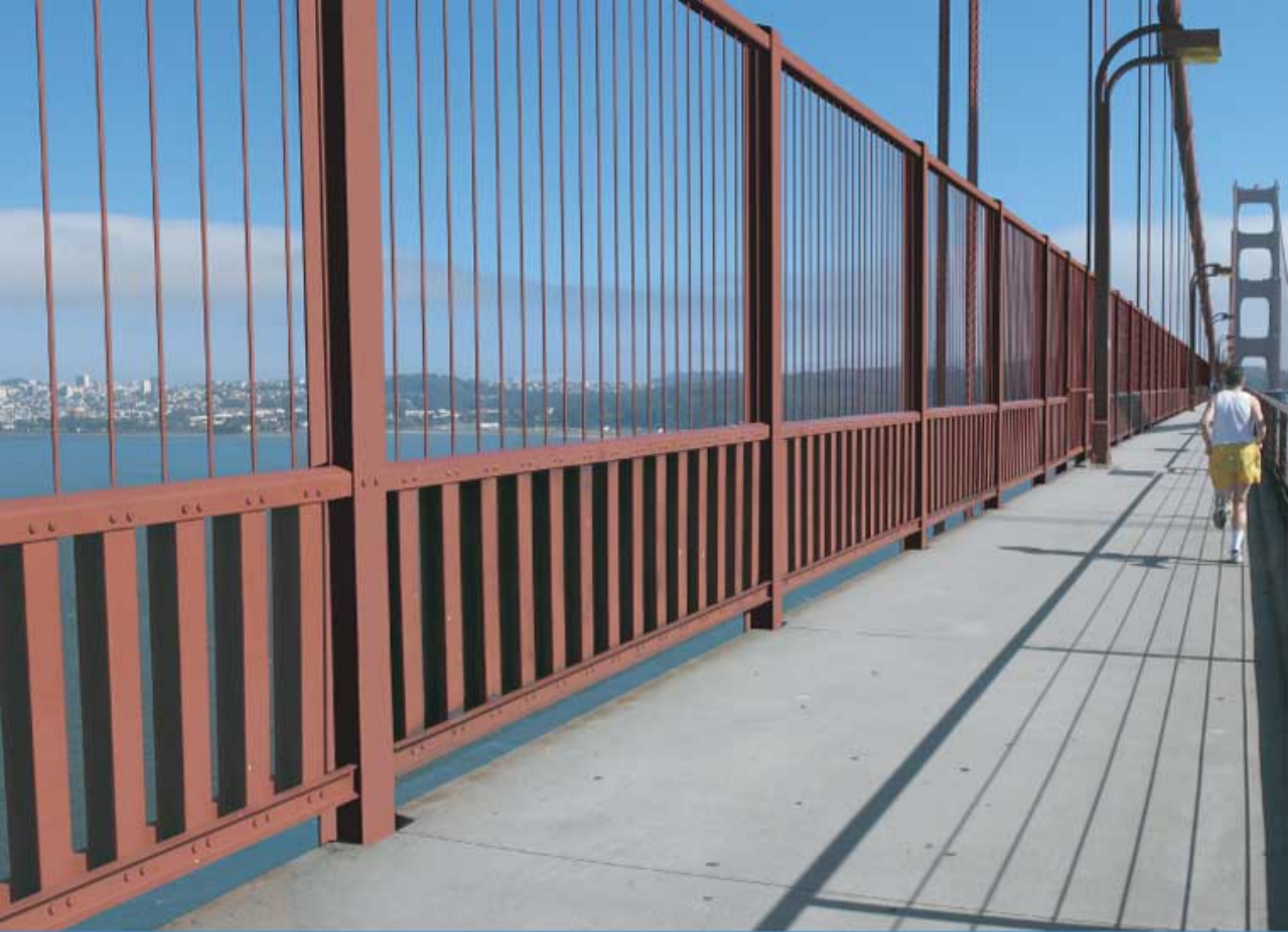
Alternative 1A - Adds 8-foot-tall vertical system to 4-foot handrail Sidewalk View South
