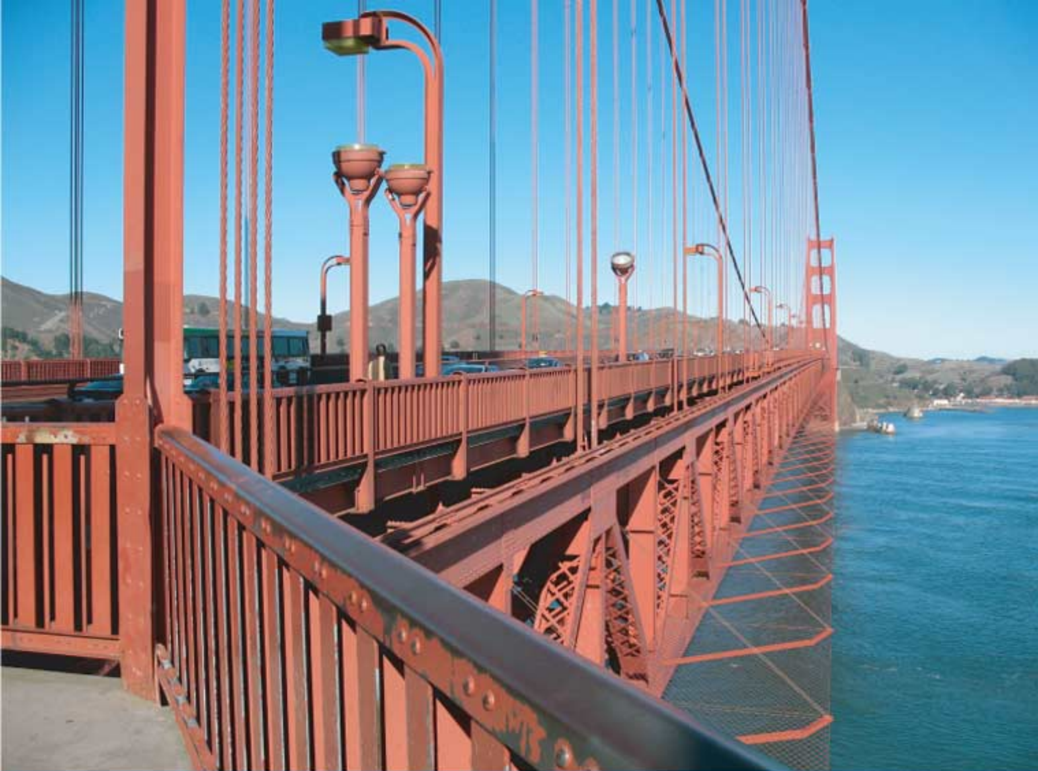
Alternative 3 - Add horizontal net system, 20 feet below and extending 20 feet out View North at Tower
