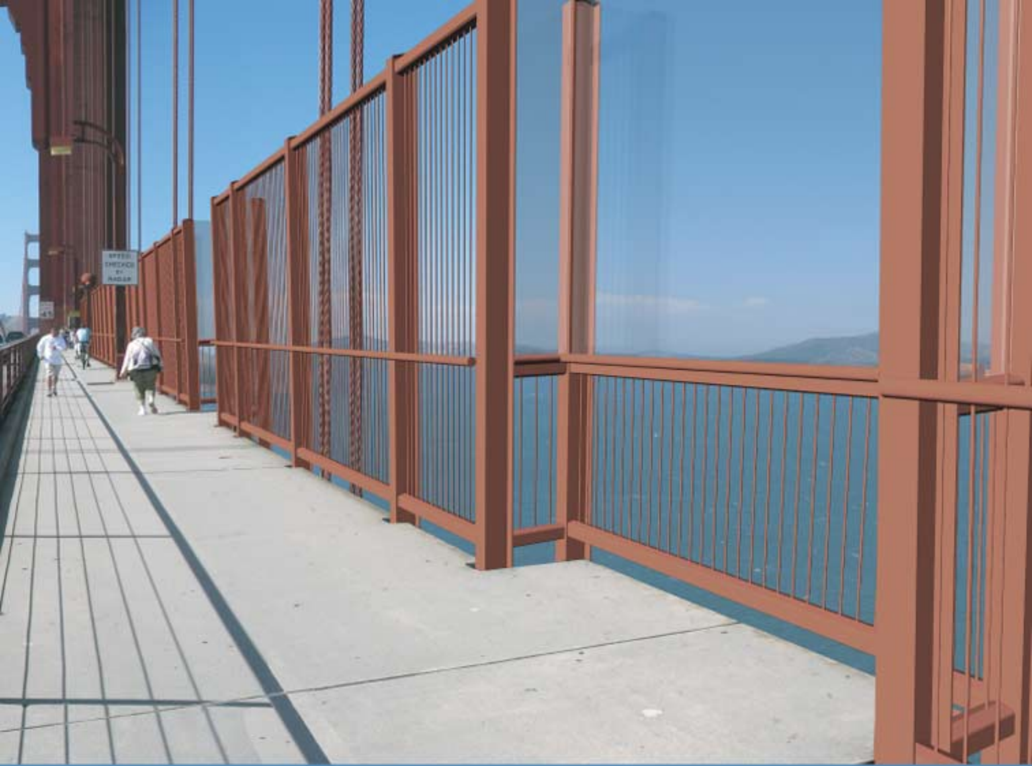
Alternative 2A - Replaces 4-foot handrail with 12-foot-tall vertical system Sidewalk View North
