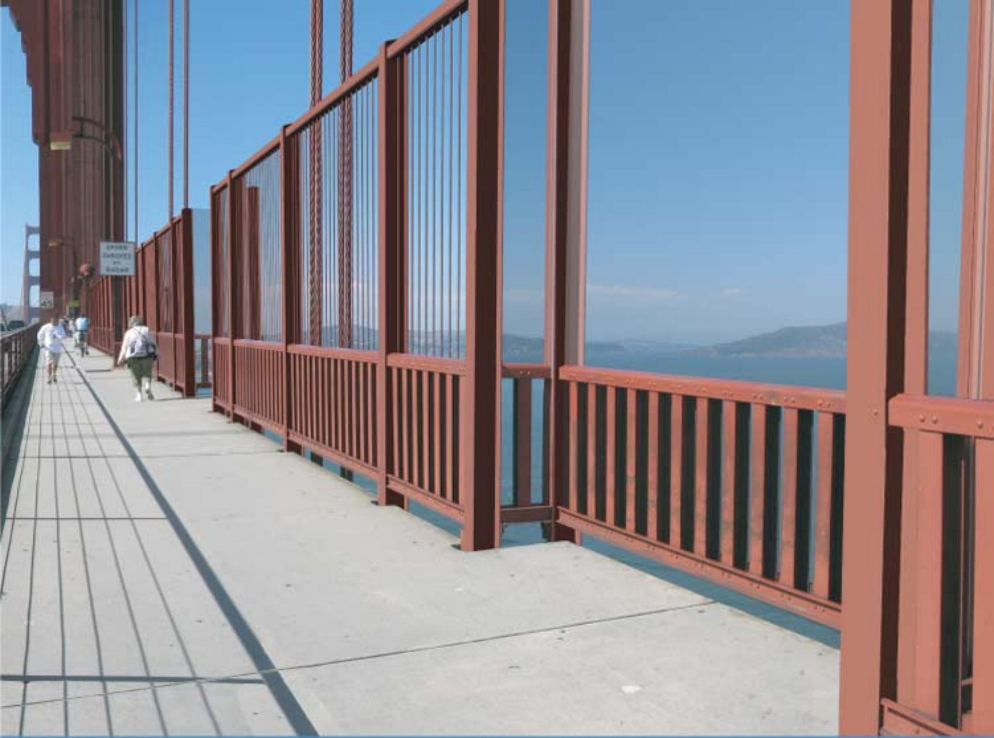
Alternative 1A - Adds 8-foot-tall vertical system to 4-foot handrail Sidewalk View North
